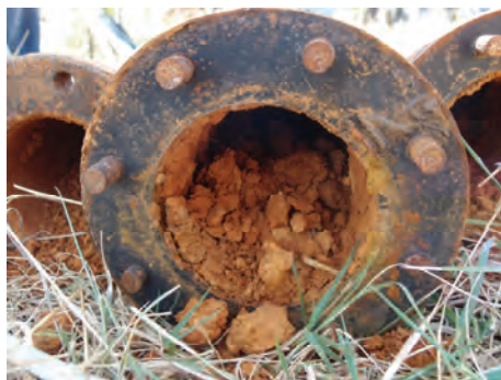
Fig. 2. Encrustations in a discharge pipe of Well Bn-6 at the water supply source of Trnovče (picture taken on 1 Sep, 2011).
